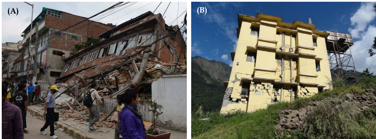
Figure 29: (A) Life safety hazard to building due to collapsed adjoining structure; (B) Life safety hazard to buildings downslope due potential sliding or collapse of heavily damaged uphill building
