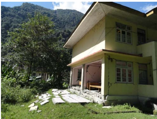
Figure 33: Extensive cracking in the infill masonry panels and out-of-plane collapse of some infill panels in an RC structure
