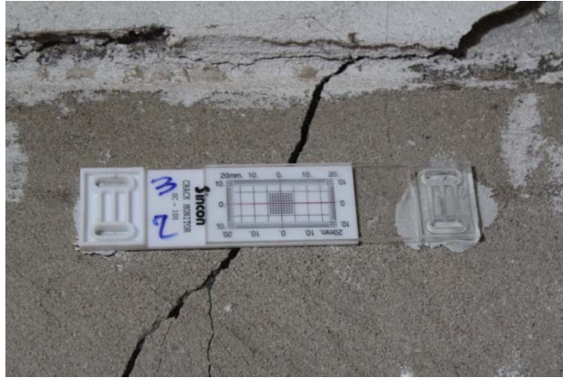
Figure 12.129: Quantitative monitoring of damaged locations with crack-width gauge
