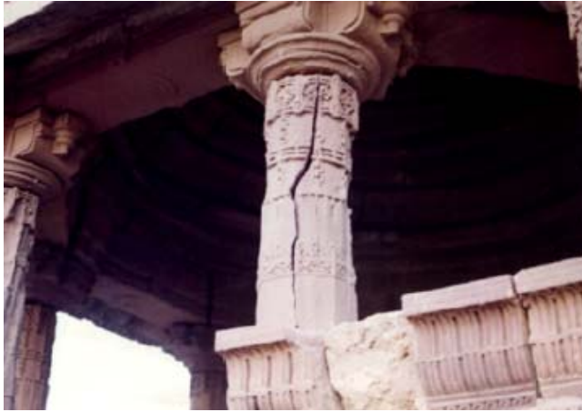
Figure 23: Splitting crack in the stone column and crushing at the base
