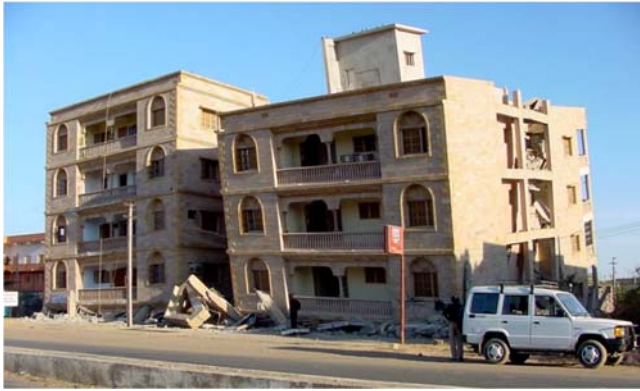
Figure 30: Failure of ground storey columns in an open ground storey building
