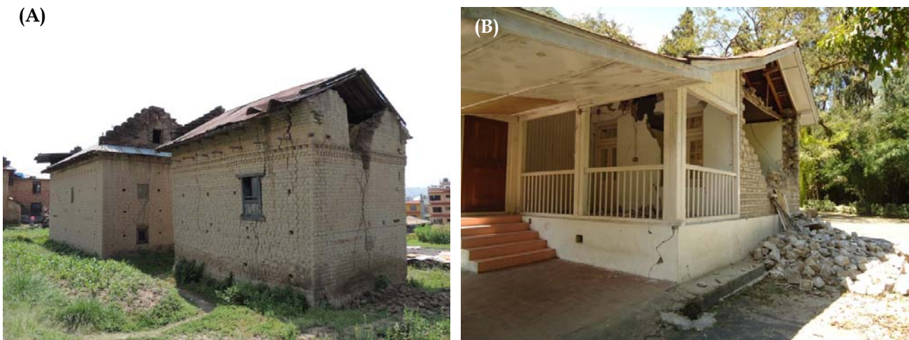
Figure 16: (A) Building showing a gable wall that has partially collapsed inwards with heavy debris loading the floor and posing a threat to the structure; (B) A building showing outwards collapse of the gable wall, leaving the supported roof system and return walls further vulnerable
