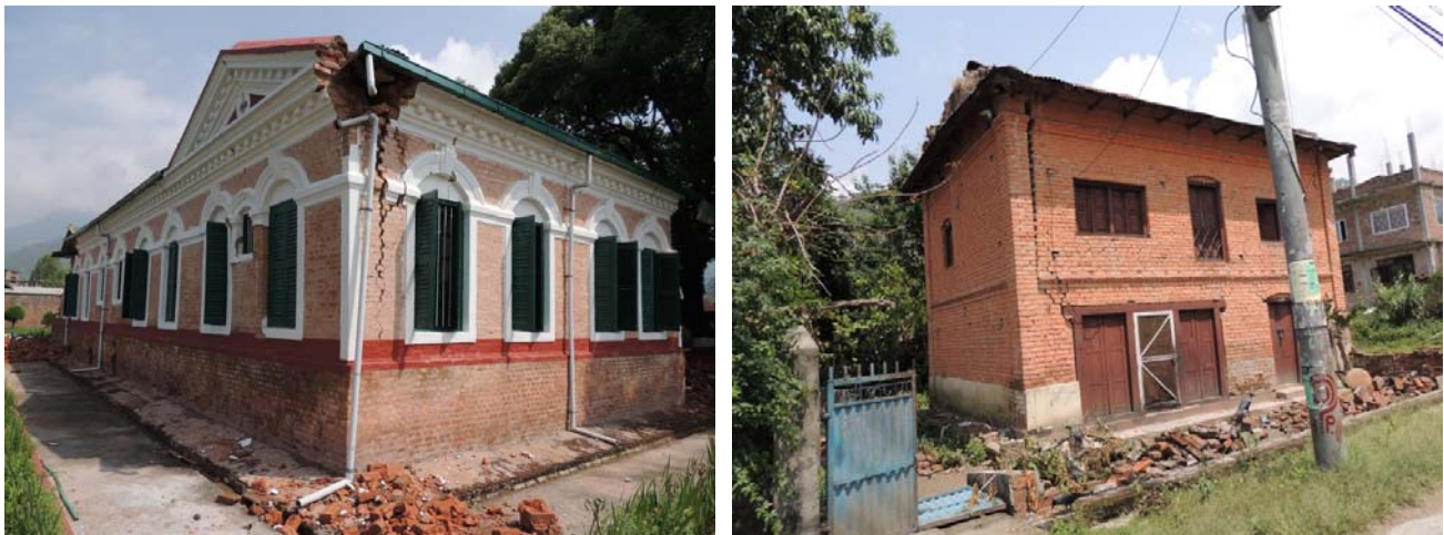
Figure 14: Buildings showing separation at the corners of perpendicular walls and out-of-plumb walls
