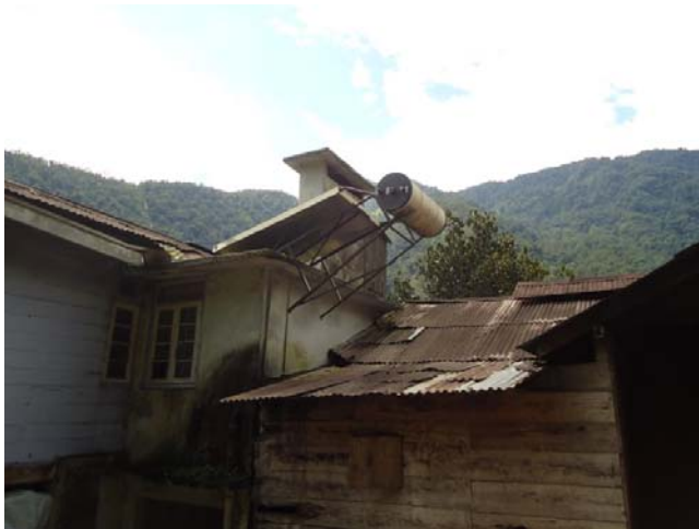
Figure 39: Overturning or dislodging of overhead water tank
