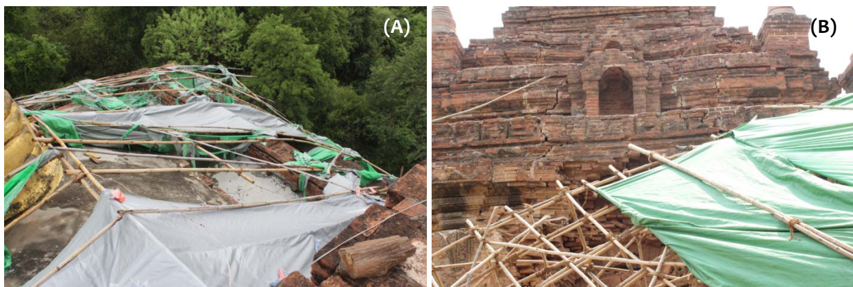
Figure 9.2: (A) Deterioration of Bamboo and Tarpaulin Sheets; (B) Wind Effect on Scaffolding
