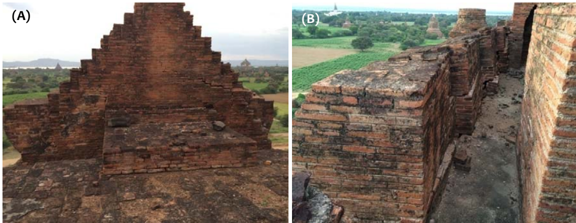
Figure 3.4: (A) Detachment and overturning of the free-standing pediment; (B) Detachment and overturning of parapet walls along the stairway
