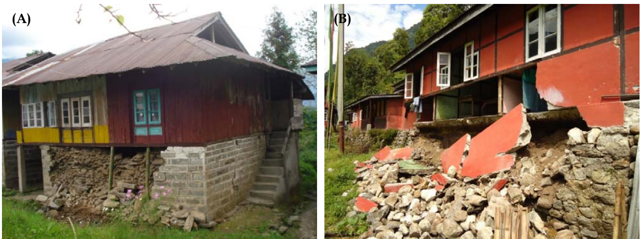
Figure 18: (A) Tilted structure due to partial collapse of RR masonry plinth; (B) Partial collapse of the structure due to disintegration of the RR masonry plinth of the structure
