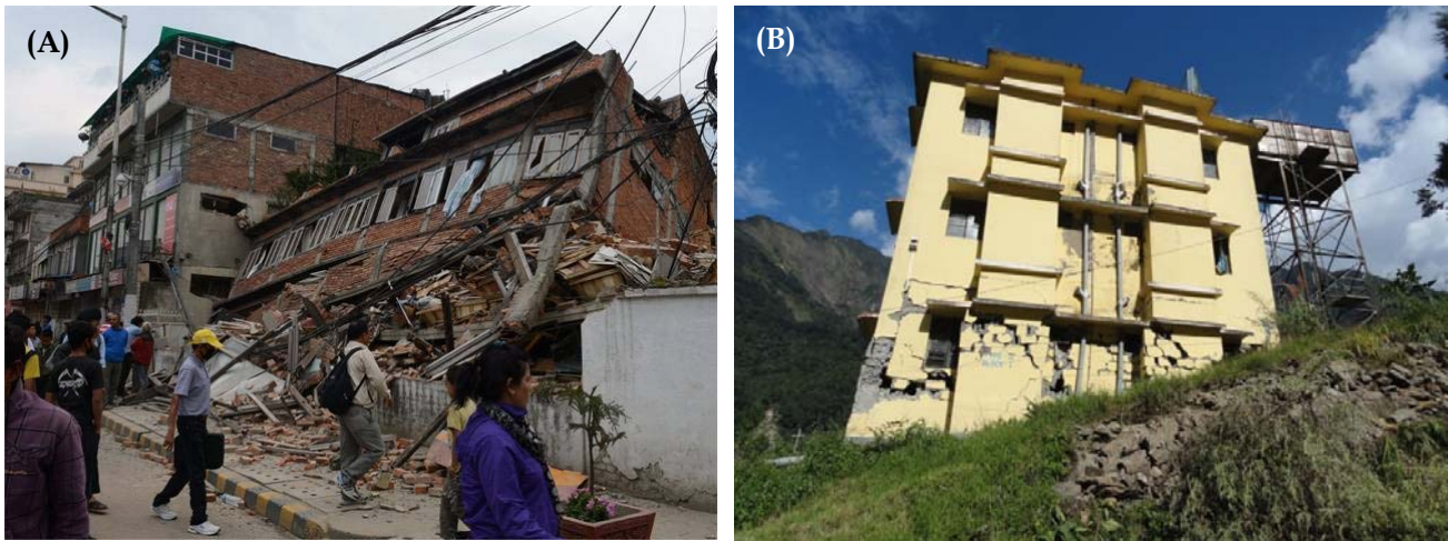
Figure 13: (A) Life safety hazard to building due to collapsed adjoining structure; (B) Life safety hazard to buildings downslope due potential sliding or collapse of heavily damaged uphill building
