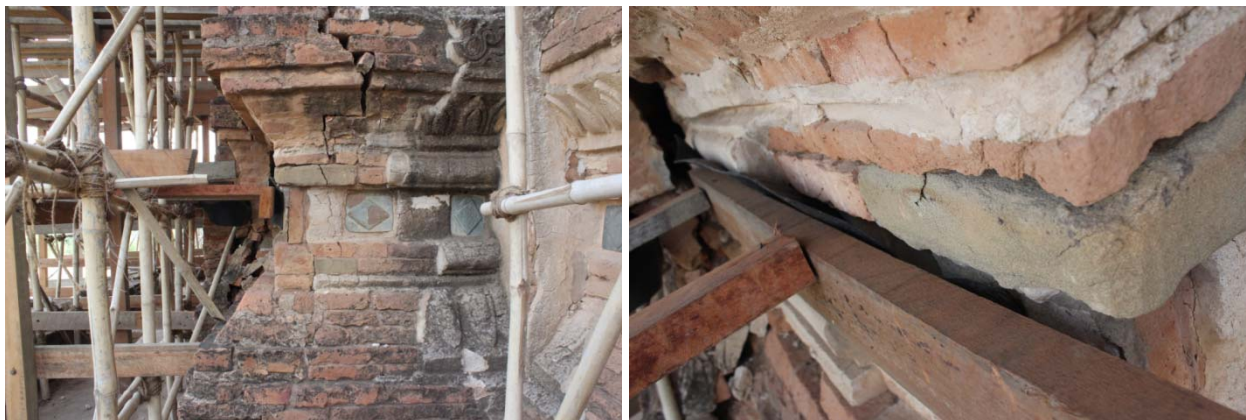
Figure 12.41: Potential hazard posed by wooden scaffolding and temporary propping members to glazed tiles
