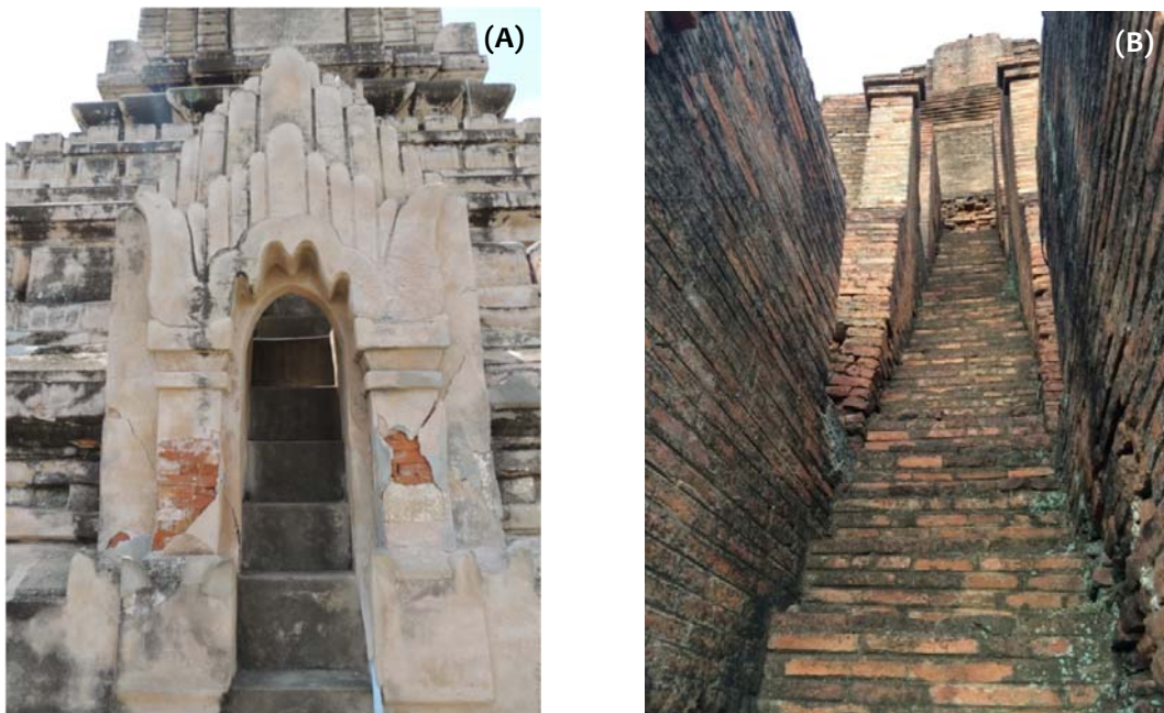
Figure 3.5: (A) Shear cracking at the supports of the entrance structure to the stairway; (B) Overturning of parapet walls along the stairway
