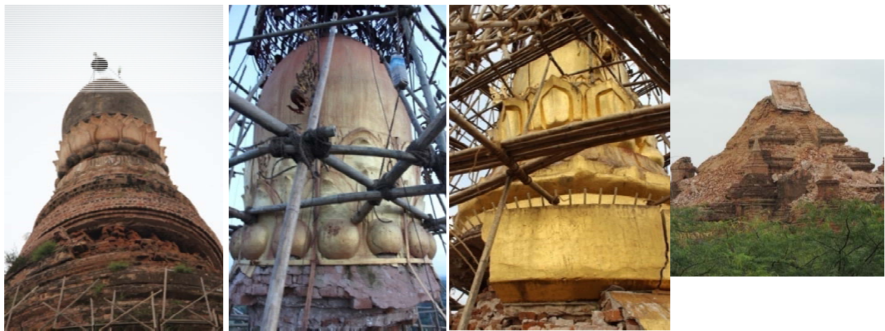
Figure 8.1: Structures with Heavily Damaged Portions Requiring Careful Removal
