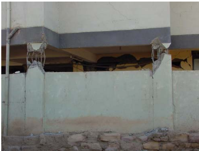
Figure 32: Shear failure in RC short columns, created due to the partial height infill panels in the RC frame
