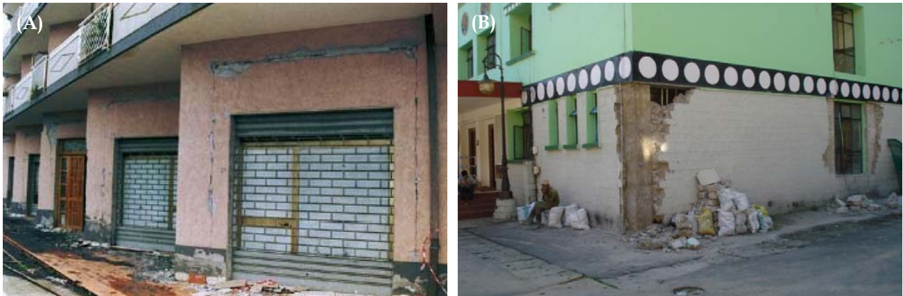
Figure 38: (A) Infill-frame separation in an RC frame; (B) Infill damage alone
