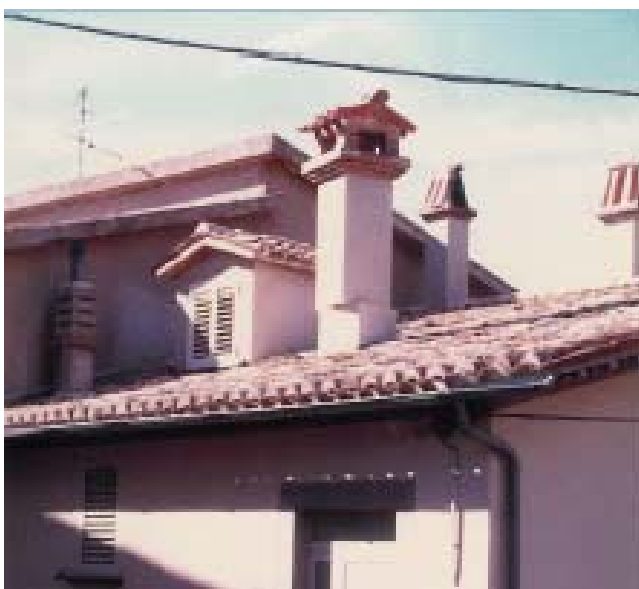
Figure 24: Damage to the chimney (a non-structural component) of the building, posing a serious falling hazard
