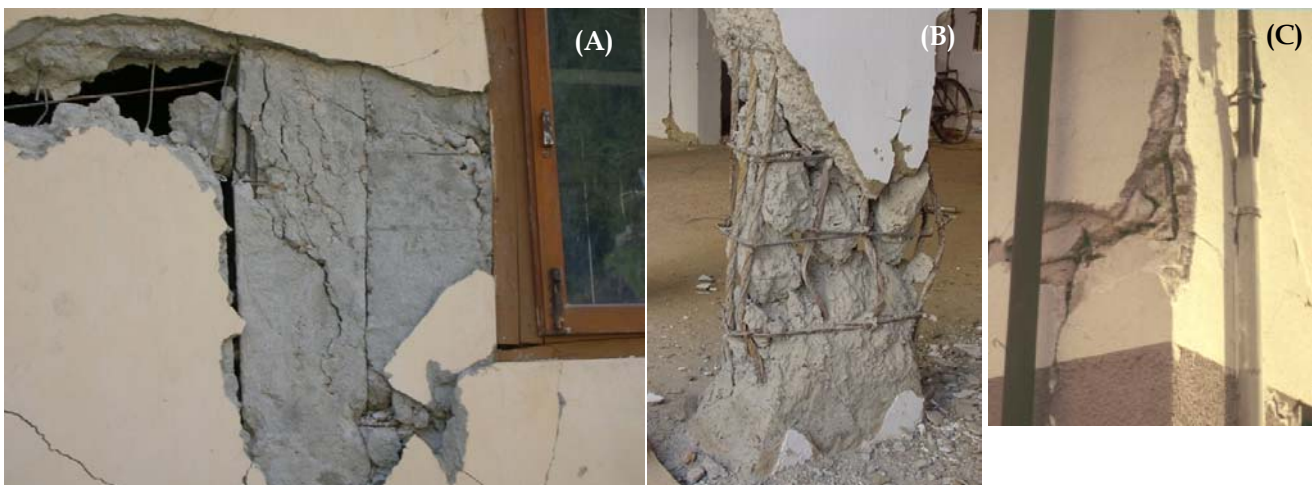
Figure 35: (A) Inclined cracks and spalling of cover concrete; (B) Inclined failure plane with spalling of concrete, crushing of core concrete, snapping of ties (note 90° hooks in stirrups) and buckling of longitudinal bars, (C) Inclined failure plane with spalling of concrete, crushing of core concrete and buckling of longitudinal bars
