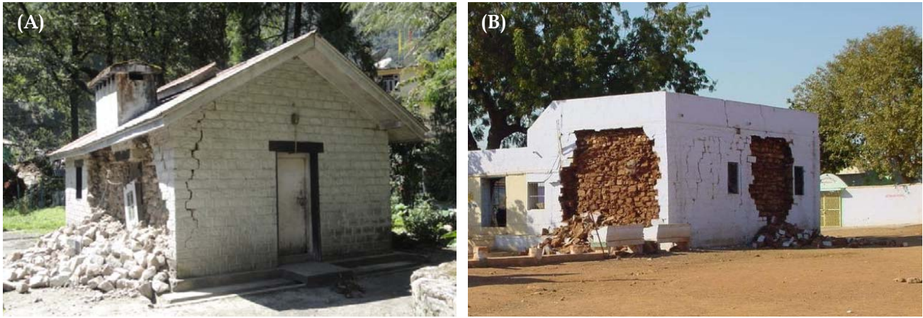
Figure 17: Separation and collapse of the external wythe of the multi-wythe wall
