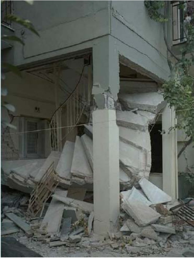
Figure 34: Collapse of the staircase of an RC frame structure with shear damage to the columns
